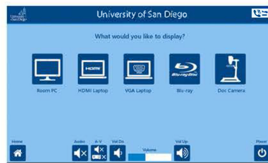
A typical control panel
